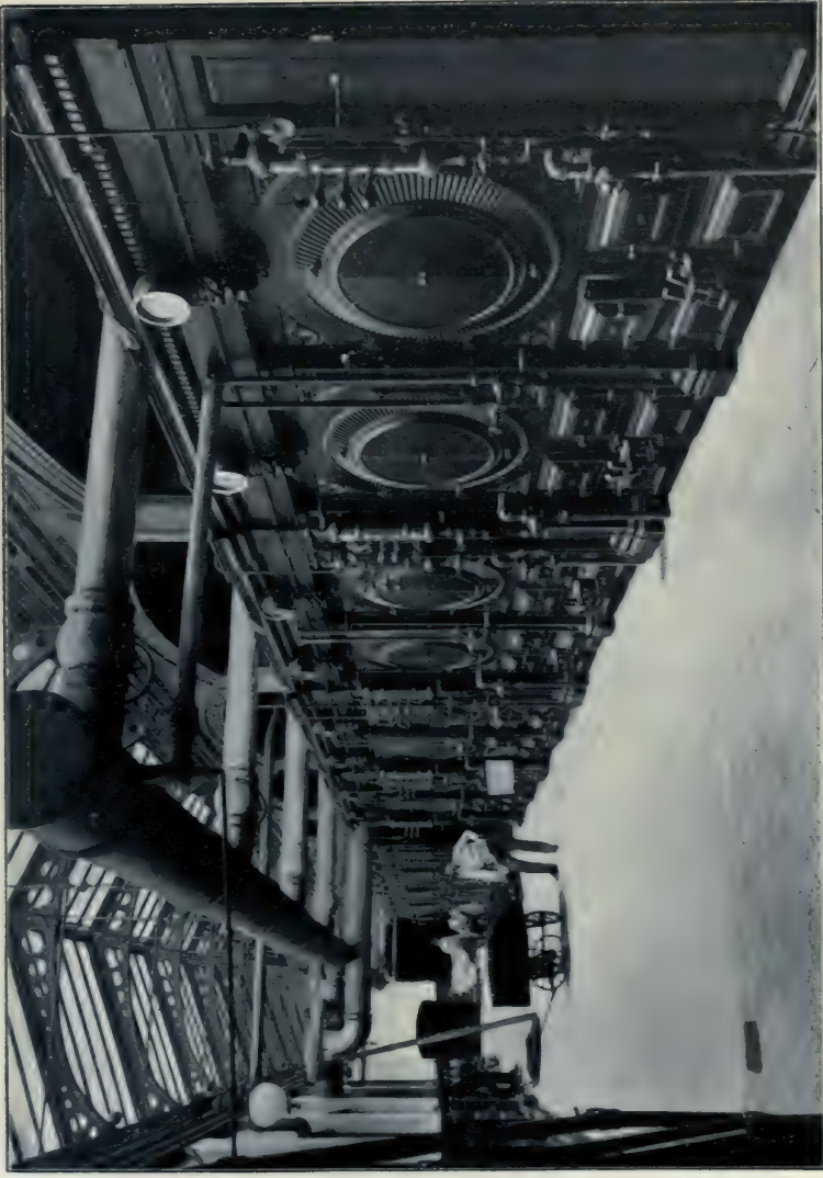
BOILER ROOM. OUTSIDE OF CELLAR AT ROOM L 1 OF PLAN.
